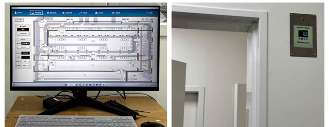
Figure 14. Automation air-control facilities
