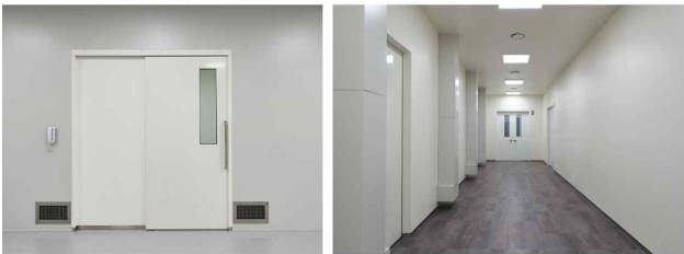
Figure 12. Convertible grill diffuser grill and duct at hall-1
