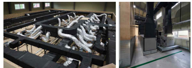
Figure 10. Simulator air conditioning facility
