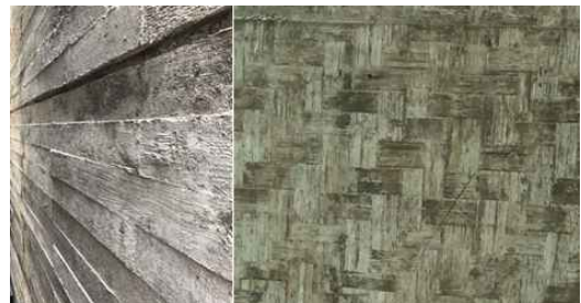
Figure 10. Liu Jiakun, Luyeyuan Stone Carving Museum, Skin made by Traditional Craftsmanship, 2001-02 : a) Skin of Wall ; b) Ceiling. (Source: taken by myself)
